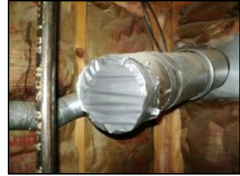
Exhaust Flue - Duct Taped
